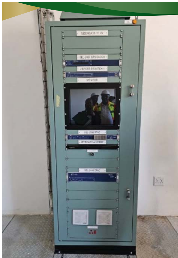
SCADA panel in Gizenga substation
