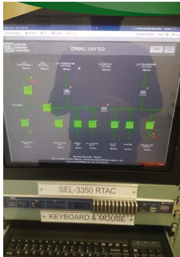
SCADA HMI screen at Zimbali substation
