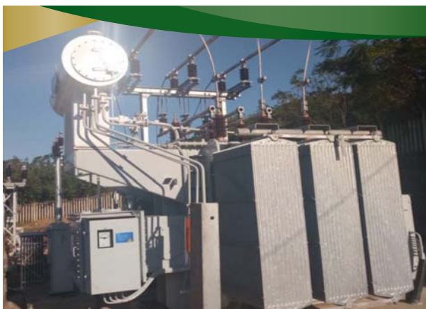
Zimballi Substation new transformer
