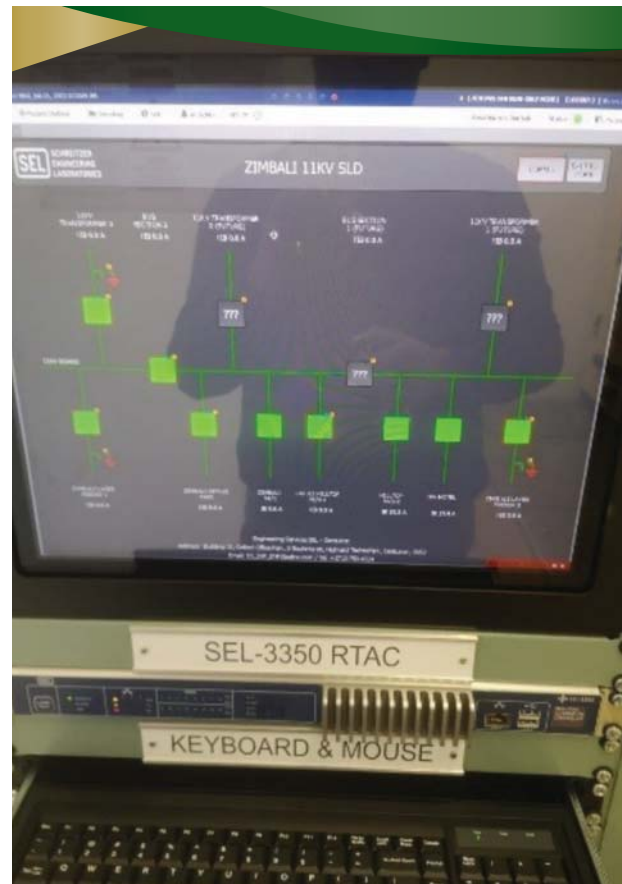
SCADA HMI screen at Zimbali substation
