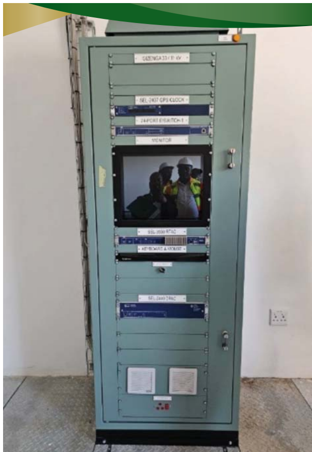
SCADA panel in Gizenga substation
