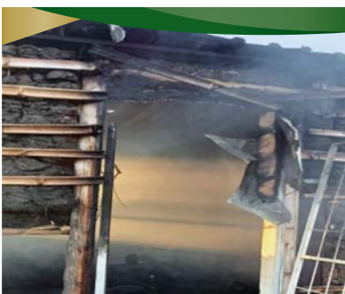
Aftermath following a structural fire incident in Ward 15 (Chris Hani) during the month of January 2023
